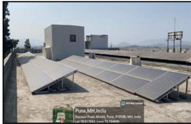
Photograph of Roof Top Solar PV Plant:
