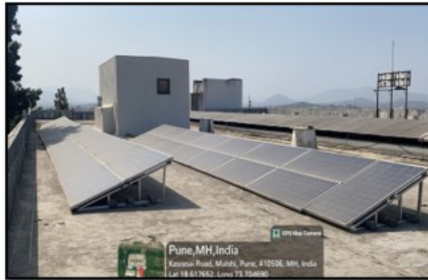
Photograph of Roof Top Solar PV Plant:
