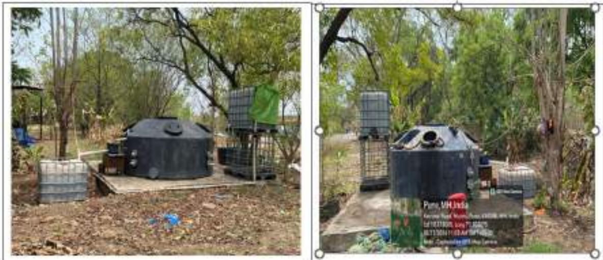
Compose Bin – Bio Gas plant
